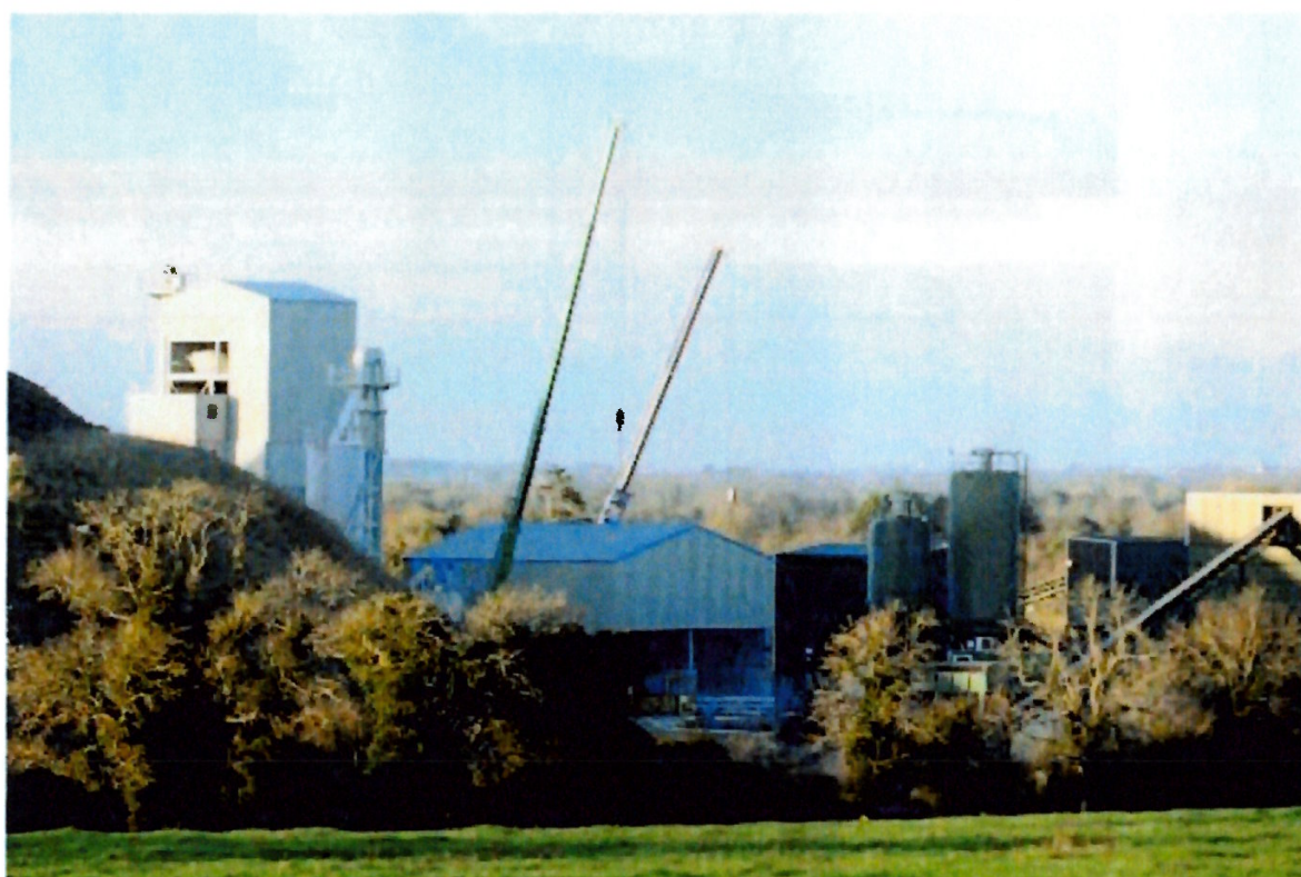
Construction of plant in 2016 without planning consent
